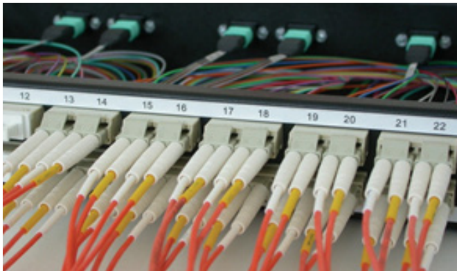
LC patch cables installed into the Starlight™ LC panel.
